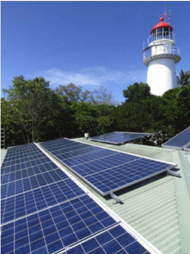
© Great Barrier Reef Marine Park Authority. Solar array 24 x 250W PV modules.
